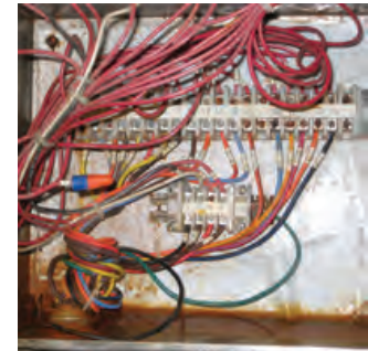
Water accumulation in electrical cabinet
