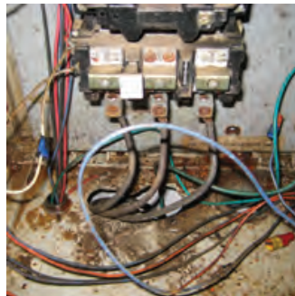
Corrosion leads to premature component failure
