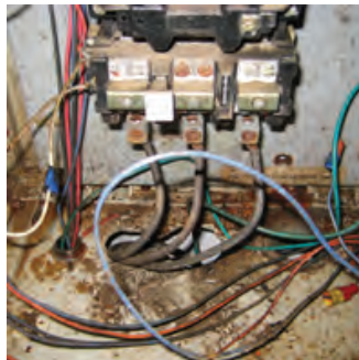
Corrosion leads to premature component failure
